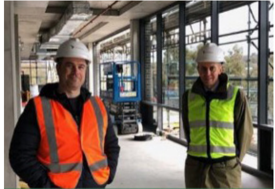
Mr Chris Leeming and Mr Andrew Kettle conducting a site inspection of T11, October 2020
